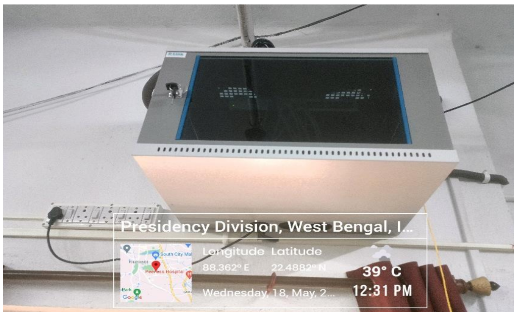
Network Switch Rack Box – Library
